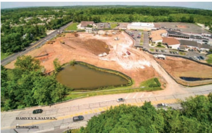
Spring House Village Shopping Center Construction Site Photo taken by Harvey Salwen on June 21, 2016.
