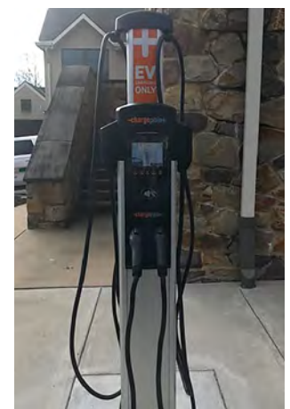
Township Building Electric Charging Station
