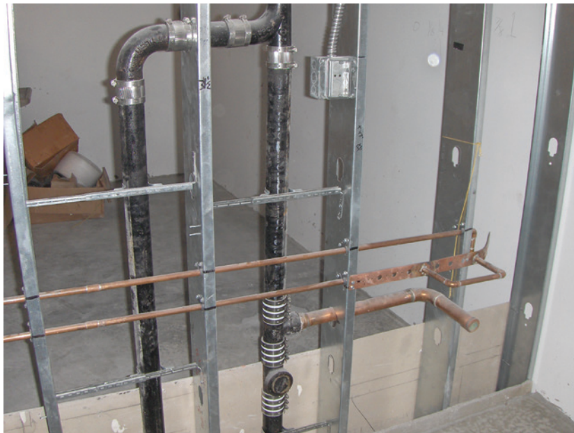
Chapter 9 of the International Plumbing Code (IPC) describes a variety of methods to vent plumbing fixtures and traps.
